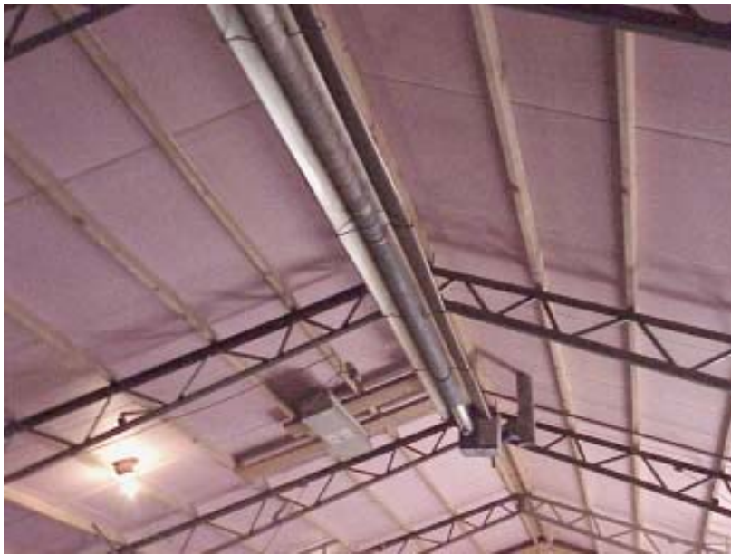
Figure1. Radiant tube heating installed in a high-ceiling poultry house. Burner unit is at far end.
