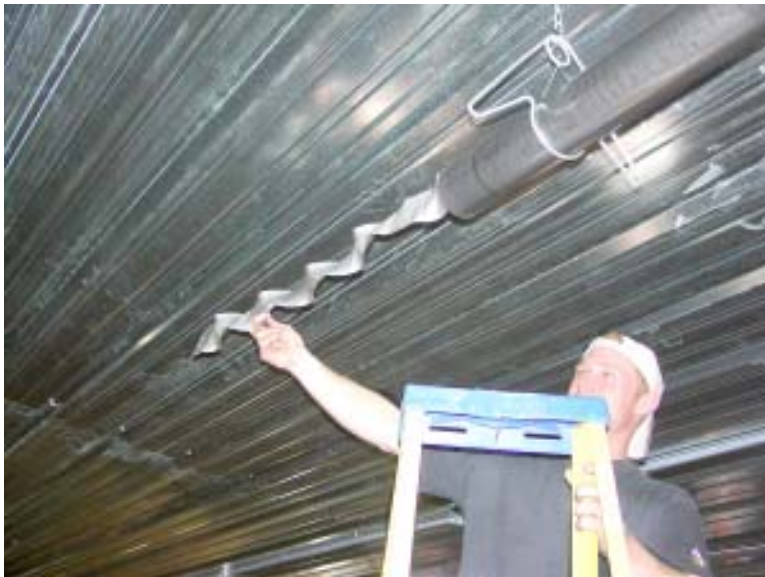
Figure 5. Workman installing element to help even out temperature from the combustion chamber to the end of the tubing. The device, installed in the last 10-15 feet of tubing, acts as a heat sink to extract heat from the exhaust gases and convert it into radiant energy. Radiant tube manufacturers use various devices of this kind to help improve the radiating efficiency of the heater. Note bracket on tubing that will be used for installing the reflector/heat shield to protect house ceiling and direct radiant energy toward the birds and the litter.
